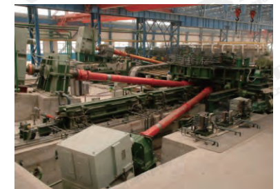
Hot Rolling Mill
